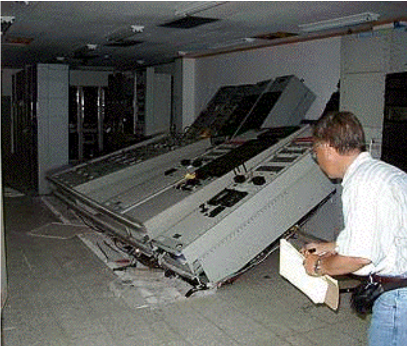
Figure 2 Toppled protective panels in the main control building of the 345 kV Chungliao substation near the epicenter of the earthquake [3]
