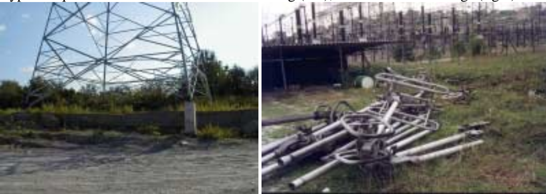
Rugged high voltage pylon (left), damage to electrical network (right)
