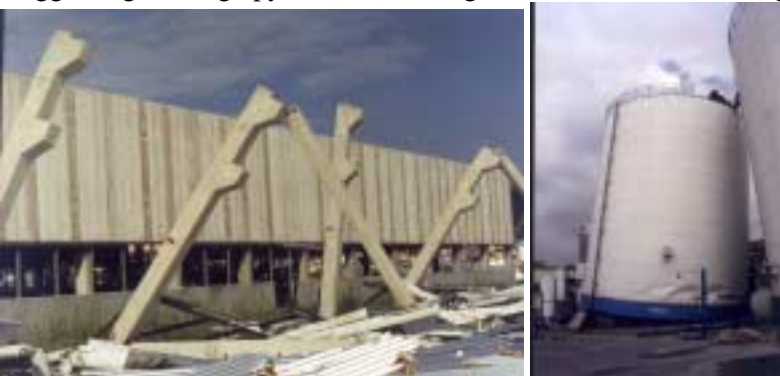
Typical precast concrete, poorly tied warehouse (left), damaged oxygen silos supports (right)
