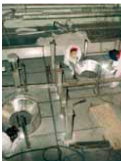
Plant improvements being implemented at the Bohunice nuclear power plant in the Slovak Republic.
