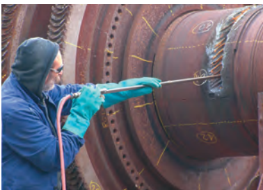
► Segmenting large plant items during the dismantling of the cooling towers for residual heat removal. Caorso nuclear power plant, Italy. [Photo: SOGIN]
