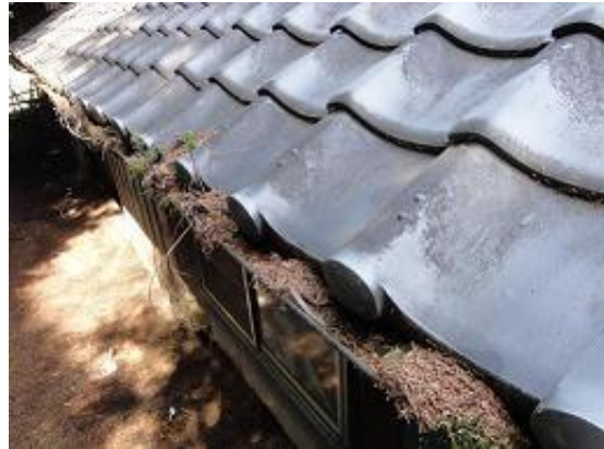
Rain water gutter (before)
