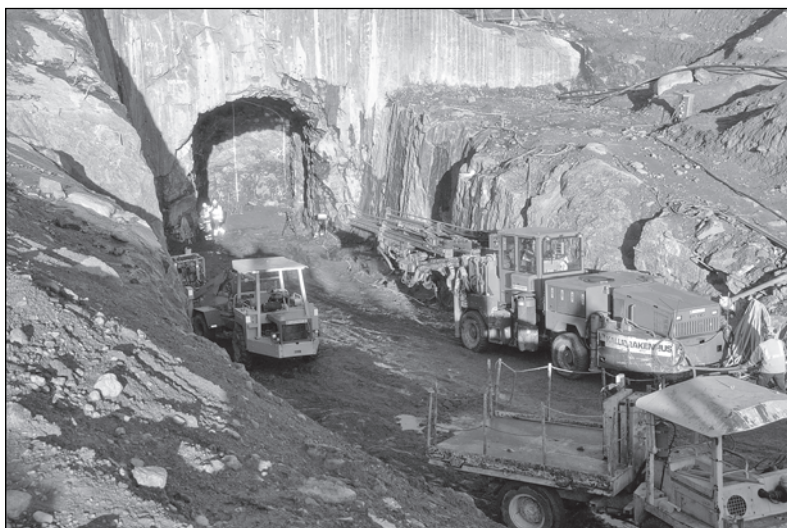
Tunnel entrance to the ONKALO underground characterisation facility at the site of the foreseen repository in Finland.
