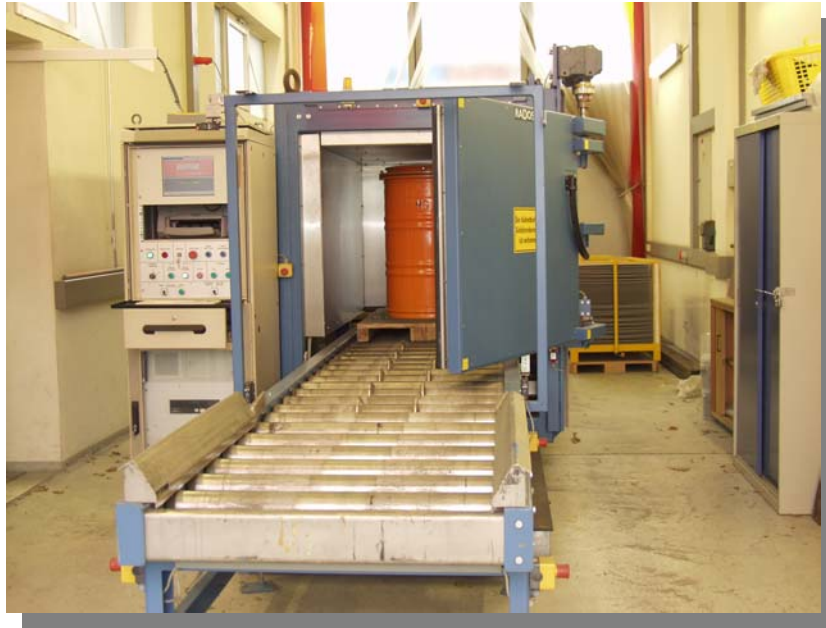
Figure 1: Release measurement facility
