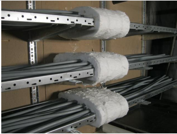
Figure 25: Wrapping of the cables by layers of mineral wool linked by a specific adhesive
